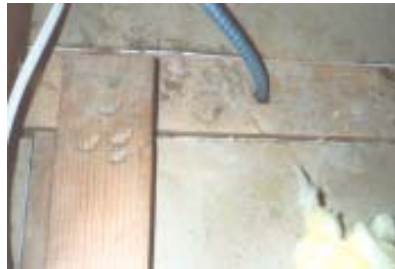
The shrunken top plate in the attic meant heated air was escaping daily during winter.
